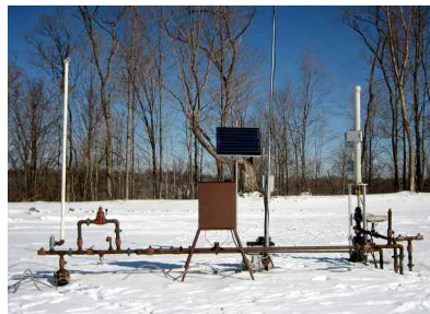
Coal-bed methane installation
